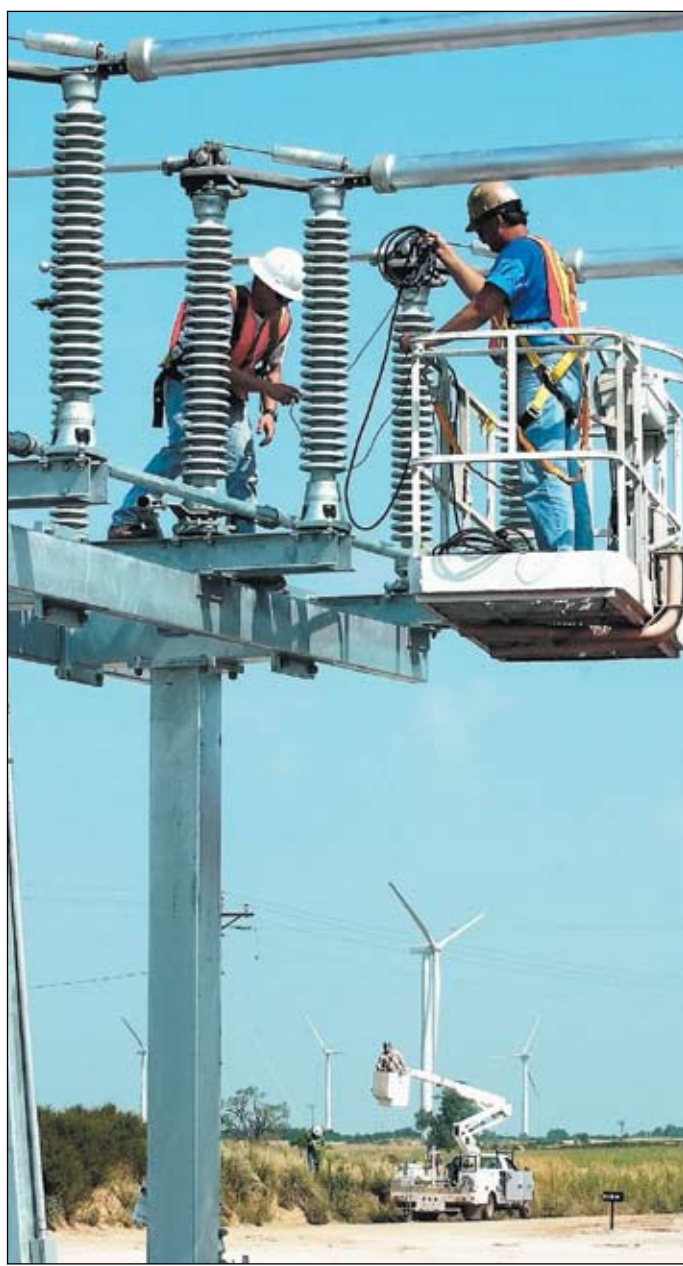
Workers assemble a substation that will carry electricity to the power grid from a wind farm near Woodward. Tulsa World file
